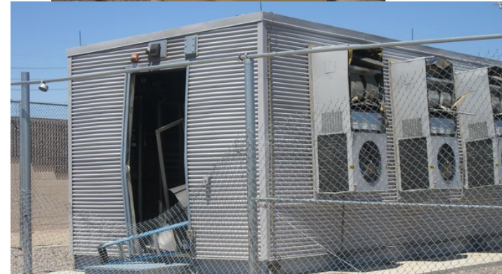
Figure 6 Damage to the rear door and HVAC systems of the McMicken BESS
